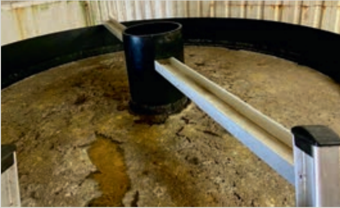
Figure 2. In this image the sludge in tank 4 can be seen. Because the active sludge was used with salt water from the RAS, the sludge is floating. Other methods to take out the sludge are needed compared to treatments for fresh water where the sludge settles at the bottom.
